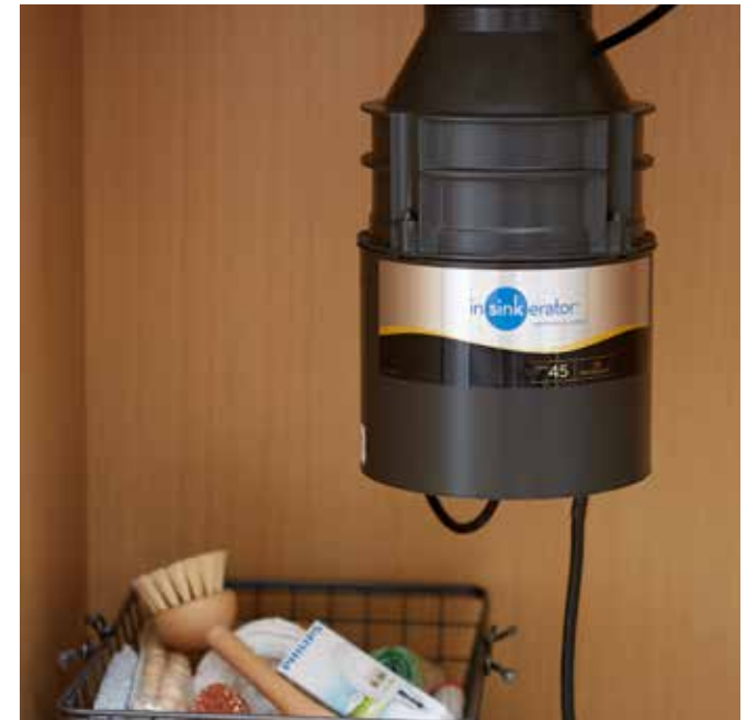
Waste Disposal Unit
